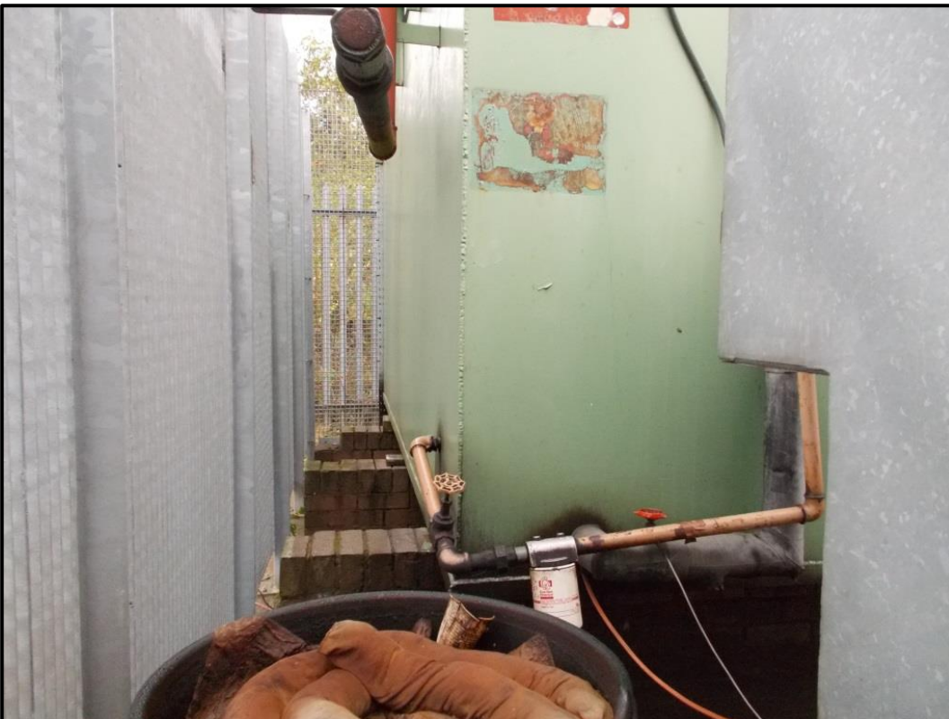
PLATE 4: STAINED SPILL RAGS LOCATED BELOW DISPENSING POINT.
