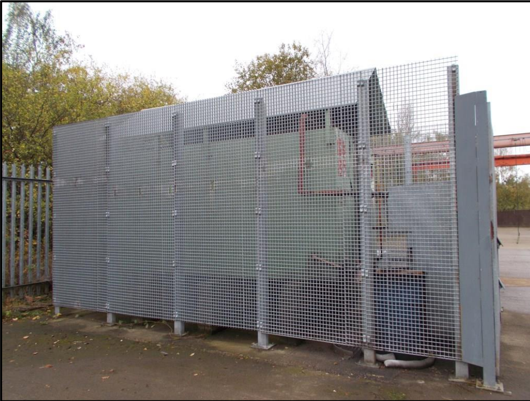
PLATE 3: ABOVE GROUND DIESEL OIL STORAGE TANK
