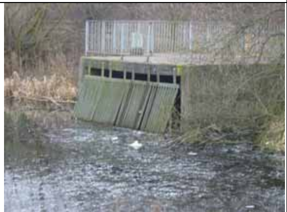
064 Trench Pool DS Overflow
