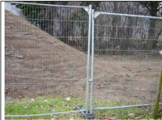
065 Hortonwood Development Site Mound of Earth Over Location of Drain
