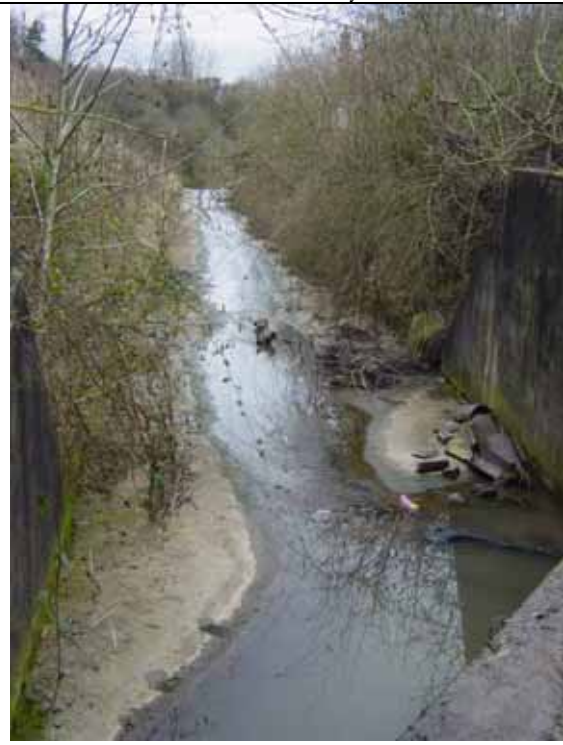
009 DS Overflow From Pool On Ketley Brook
