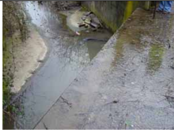
008 Overflow From Pool On Ketley Brook
