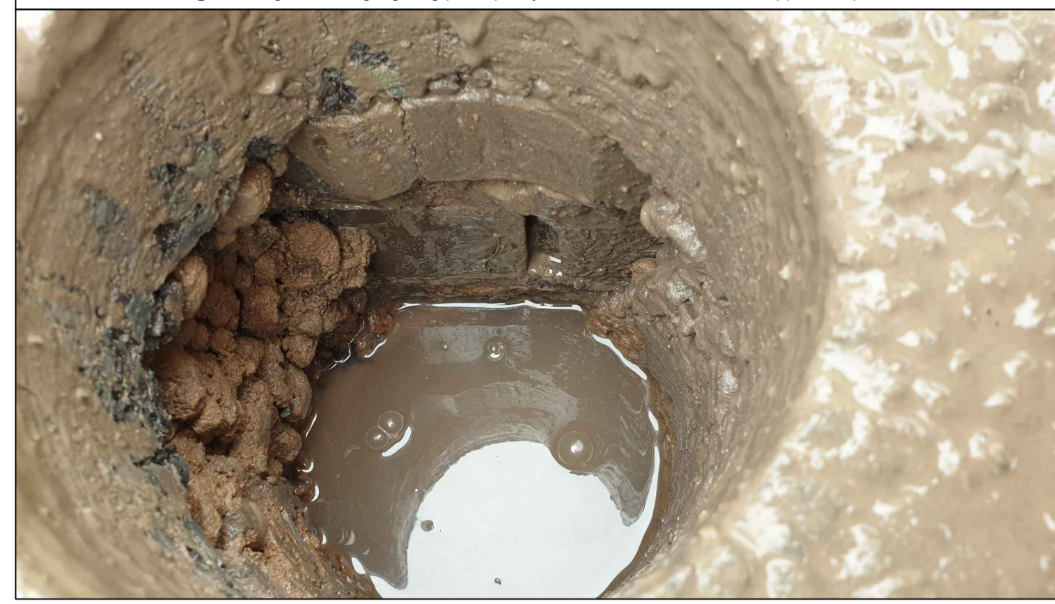
Core 2 @ Chainage 58m: Highlighting poor quality concrete and brickwork, at approx. depth 100mm
